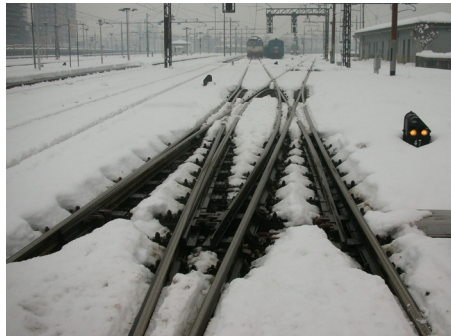
Typical Heated Points Systems Milan, Italy.
